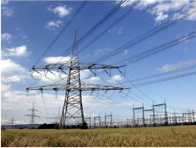
Fig 5.48 Electric power Transmission lines
