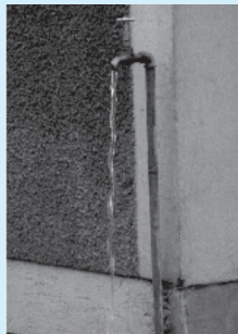
Picture 9.1. Water dropping from pipe
